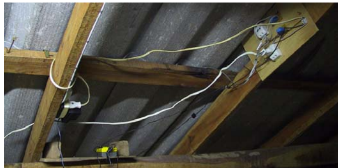
Figure 5. The switchboard in action.
